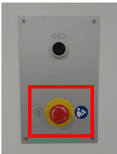
Figure 10. Emergency door release button in scanner room (indicated by red square)
