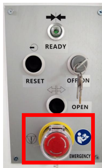
Figure 11. Emergency door release button in control room (indicated by red square)
